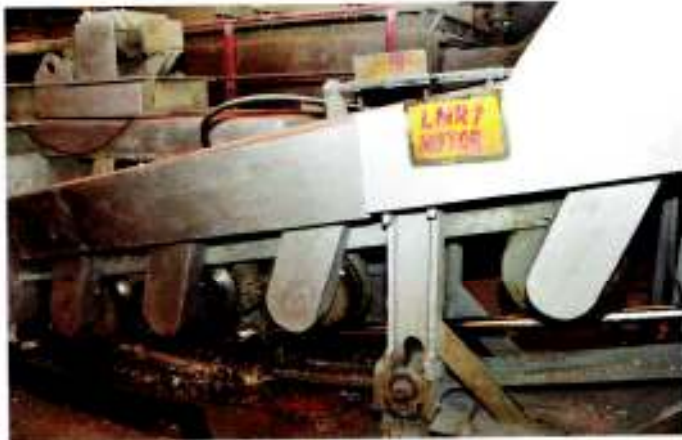
Extraction system of tubes from molten bath of zinc during hot dip galvanising of tubes
